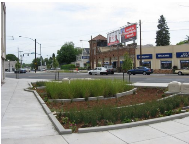
Figure 2. This bioretention area takes runoff from the street through a trench drain in the sidewalk as well as runoff from the sidewalk through curb cuts (Source: Abby Hall, US EPA).
