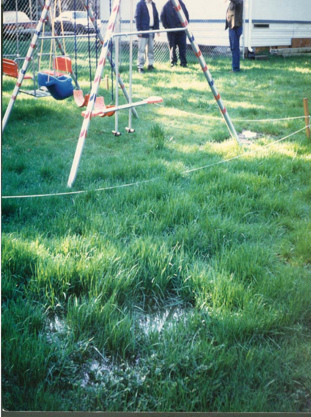
Exposed septic tank.
