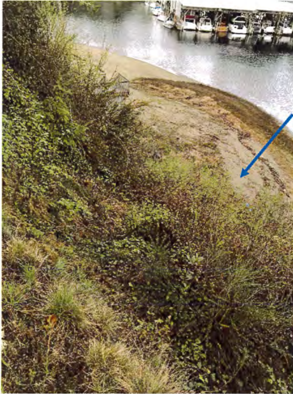
Photo #1 – Beach from the top of the Bluff. Occasional high tide or winter storms may directly impact the base of the bluff but active erosion from the toe does not appear to be the predominant cause of bluff erosion. Established vegetation is observed at the base of the bluff.
